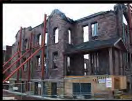
◀ Remains after devastating fire.
